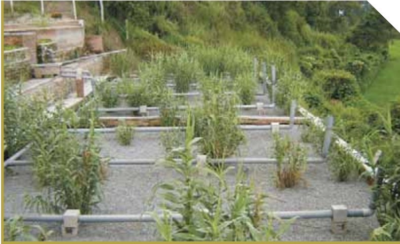
Vertical flow CW in operation and after vegetation growth
